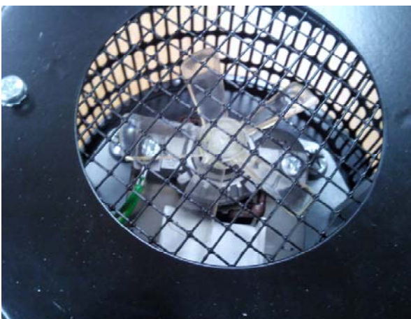
Figure 2. Original cooling fan in situ.
